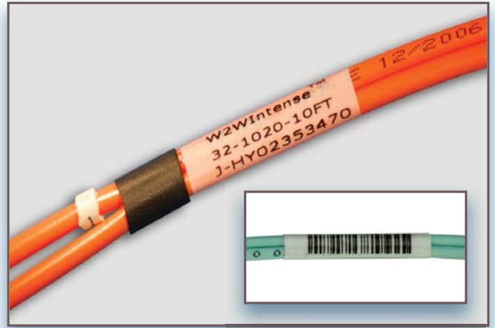
figure 4: Every cable is labelled with a serial number and a barcode (fiber only)
